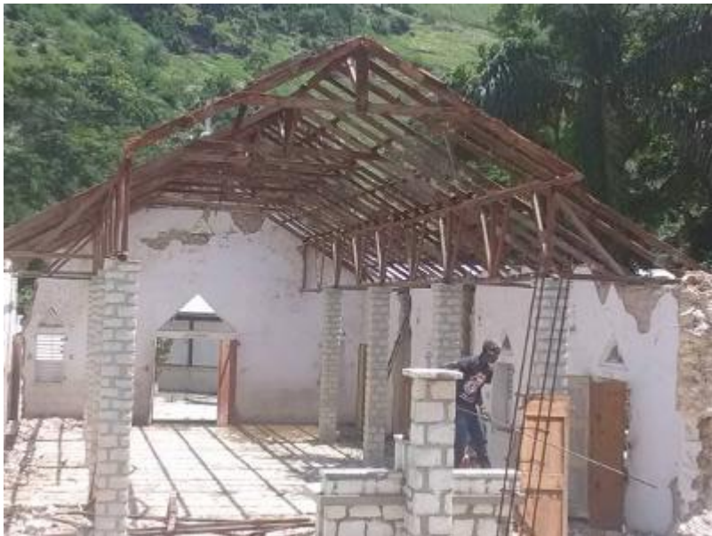
As of July of 2020, the walls and roof supports of the new church were in place. Builders are currently working on finishing the roof, but we still need more funds to complete the project.
